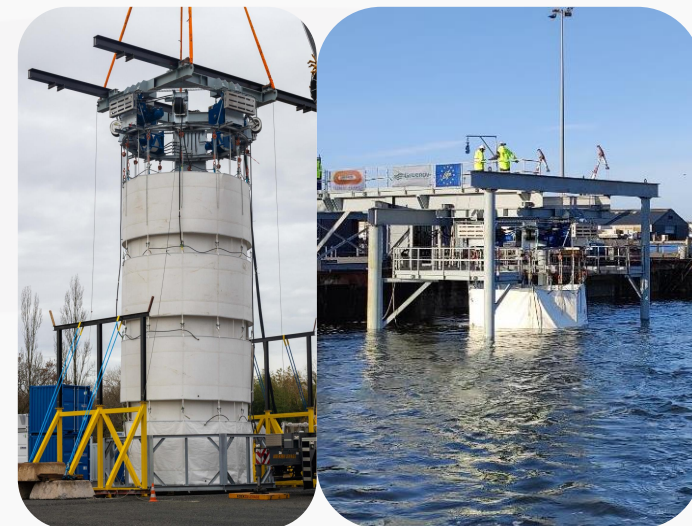
The SubSea Quieter (SSQ) Pile Driving , for a local containment dedicated for isolated pile
