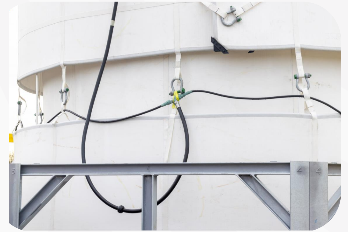
The network of piping connected to the air management systems
