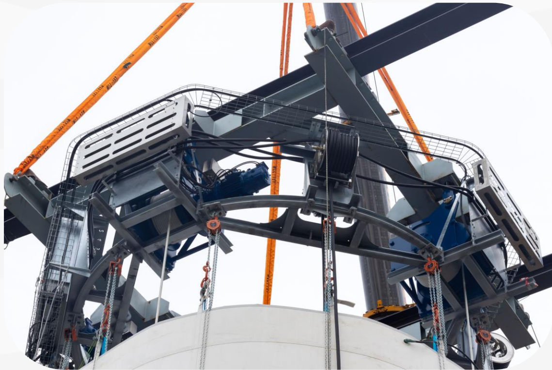
The handling system with automated winches
